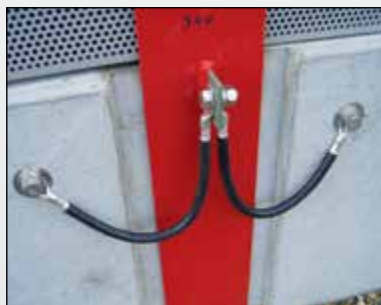
earthing terminals at base elements
