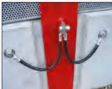
earthing terminals at base elements
